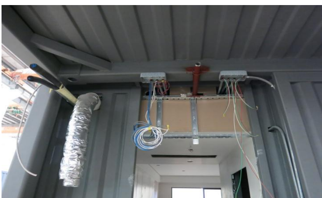
PICTURE 4: ELECTRICAL, VENTILATION AND DRAINAGE SYSTEM
